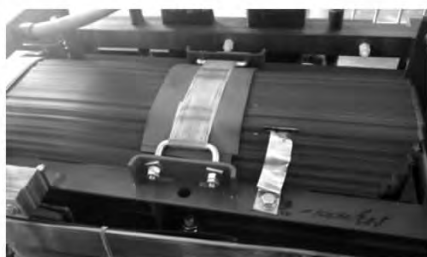
(c) 铁芯接地铜排烧断
