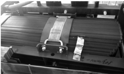
(c) 铁芯接地铜排烧断
