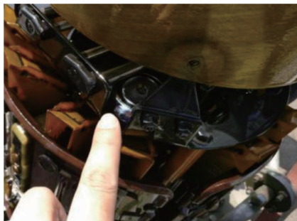
(b) 掉落的均压螺栓
